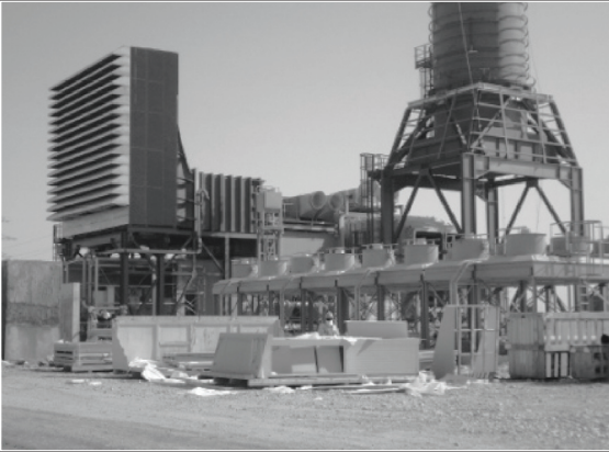
The Erbil Power Plant
